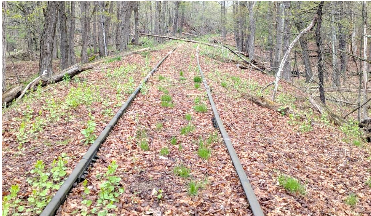
Figure 3 –Missing / Buried Ties
