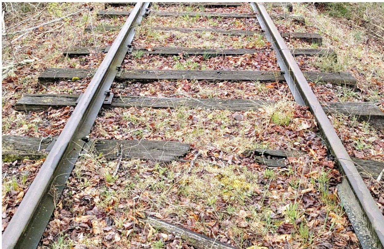
Figure 4 – Deteriorated Ties and Loosening Spikes
